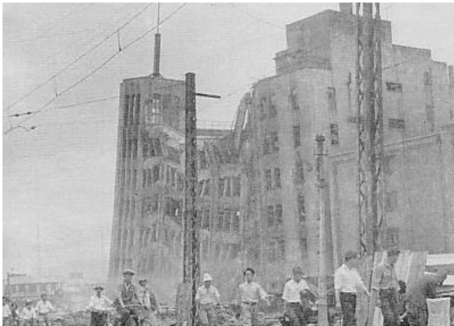
Figure 3.11. Daiwa Department Store After the Fukui Earthquake (Wikipedia.com).
