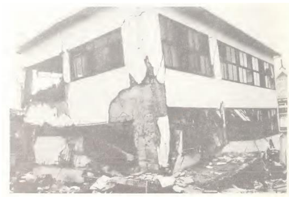
Figure 3.14. Paloma Buildings, Damage from 1978 Miyagi Ken Earthquake (Brady, 1980).
