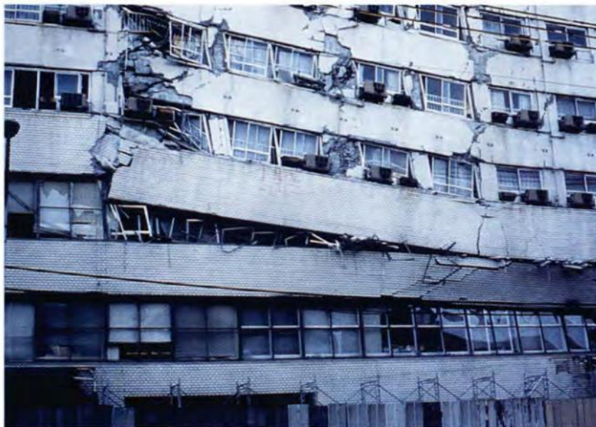
Figure 3.17. Collapsed Wooden Building and Apartment Building in 1995 in Great Hanshin Earthquake (Muguruma, Nishiyama, & Watanabe, 1995).
