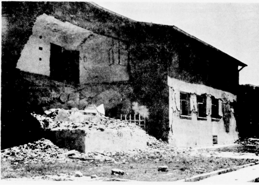
Figure 3.24. Completely Destroyed Police Building in 1975 Lice Earthquake (Mitchell, 1976).
