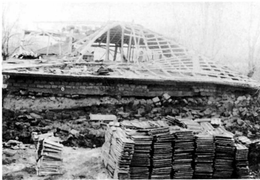
Figure 3.21. Damage from 1939 Erzincan Earthquake (William, Pomonis, Booth, & Ring, 1992).
