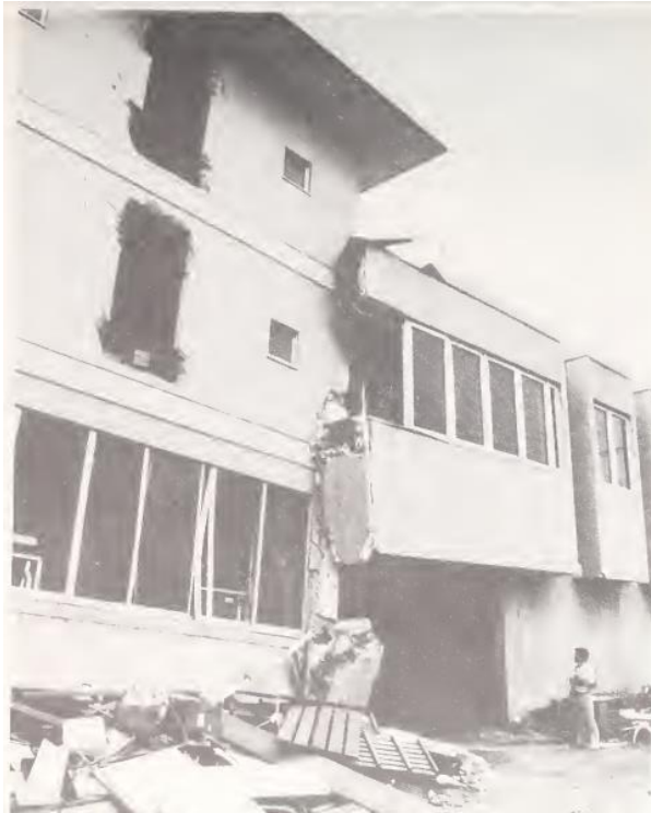
Figure 3.15. Yazaki Industries, Damage from 1978 Miyagi Ken Earthquake (Brady, 1980).
