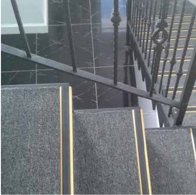
Figure 10: An Example of Surface Cover and Stabilizer on Stairs That May Cause Accidents ("Stair Covering," 2017).
