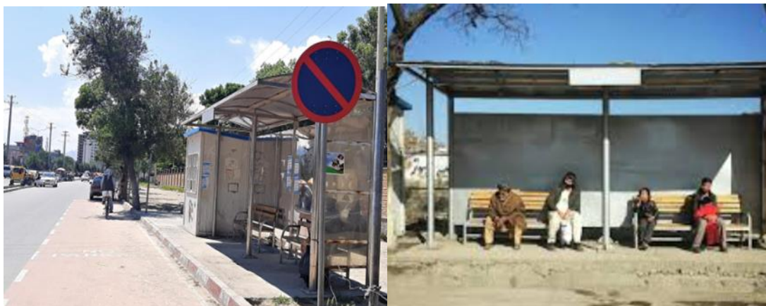
Figure 5.2. A bus stop with a shelter in a busy commercial area, showing the inadequate size and lack of maintenance.(Author, 12.05.2024)
