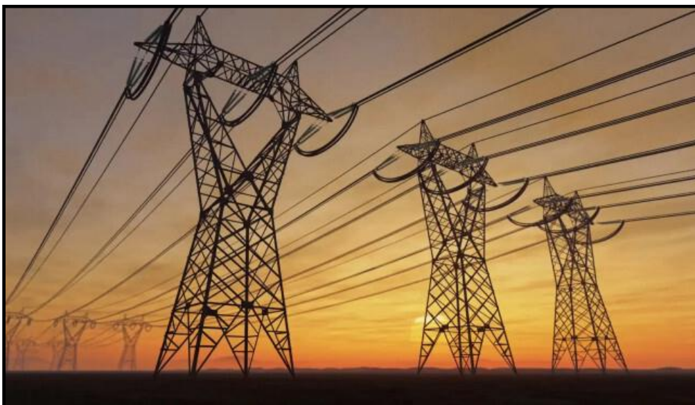
Figure 2.4. Transmission Lines (above 300 kV).
