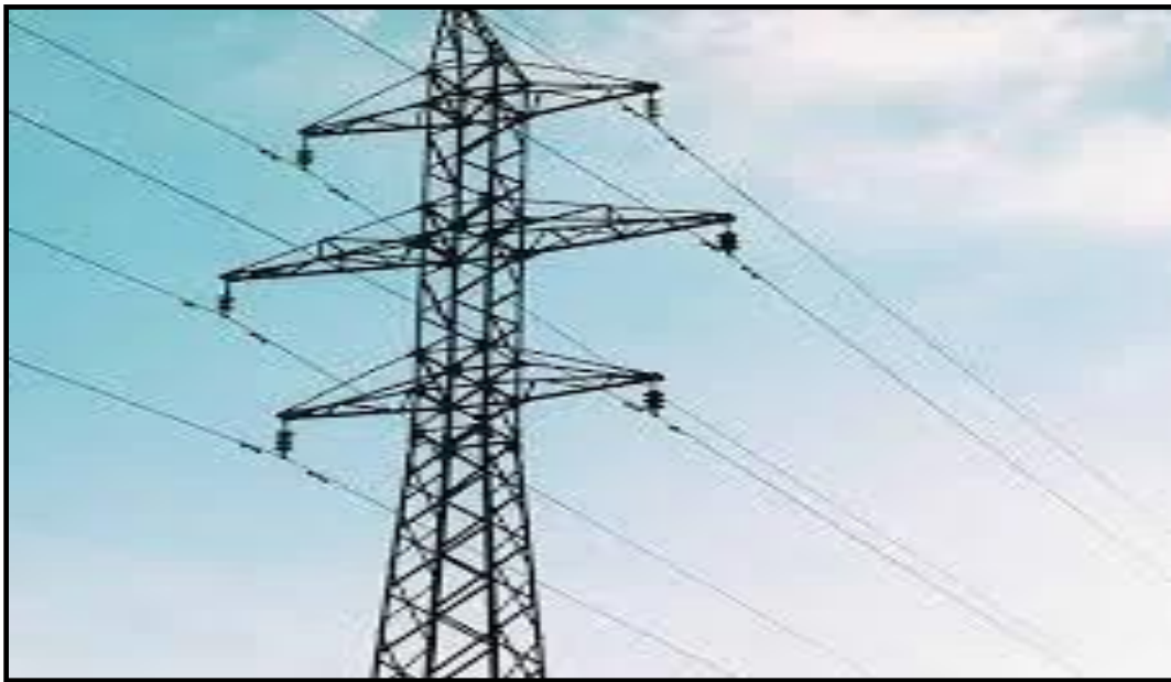
Figure 2.5. Transmission lines (33 kV)
