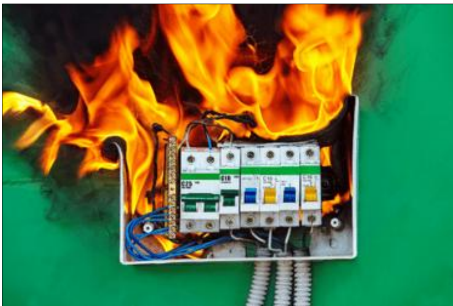
Image 3.6. Electricity leakage (URL-14)
